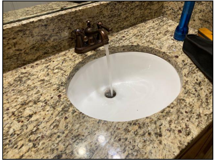
128. Sink is functional
