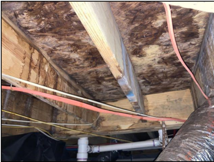
68. Large water stains under kitchen/living room
