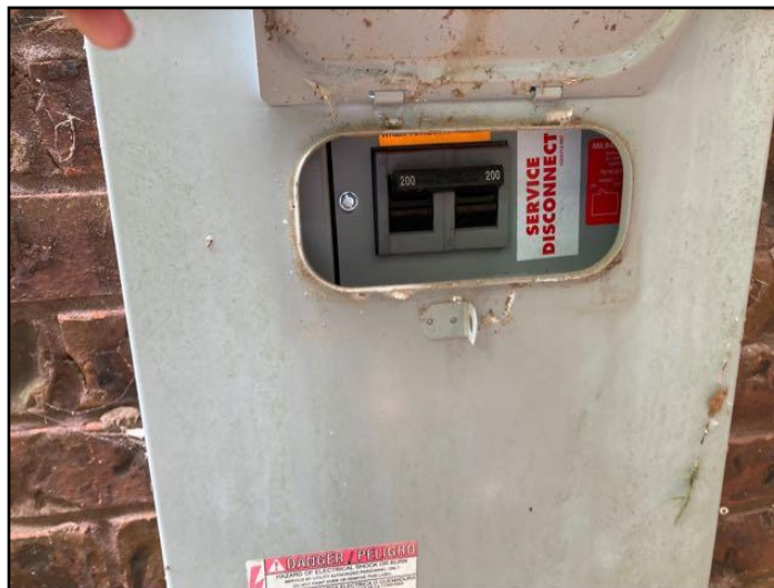
74. Main electrical shut-off
