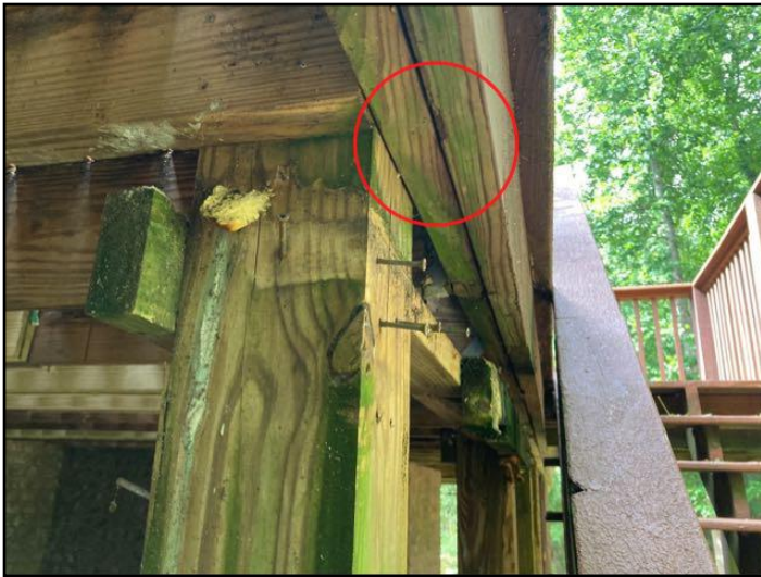
40. Improper beam connection detail
