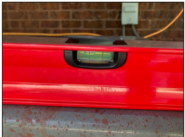
98. Condenser not level
