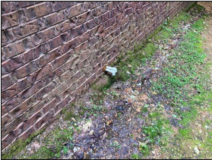
103. Condensate discharge location
