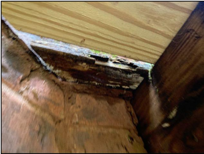
36. Rot/damage at deck edges
