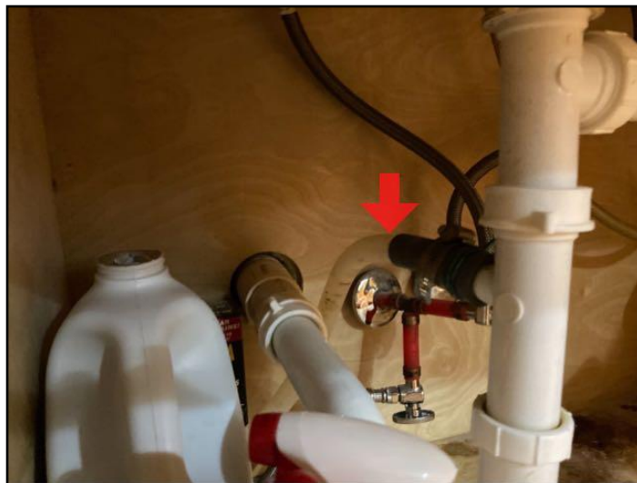
120. Backflow prevention missing
