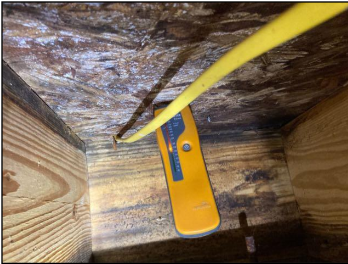
72. Borderline moisture content under laundry
