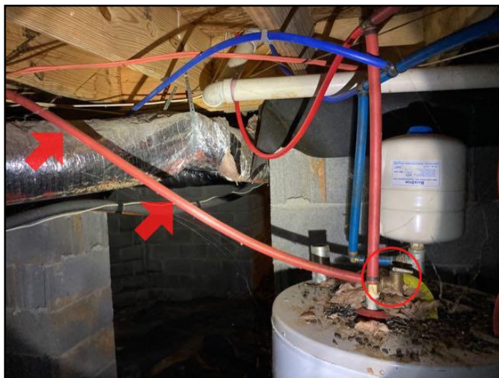
113. Improper relief valve discharge tube
