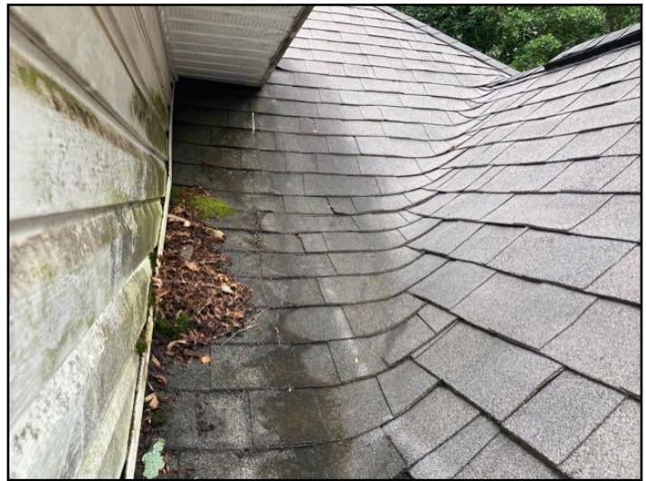
2. Debris/ moss growth
