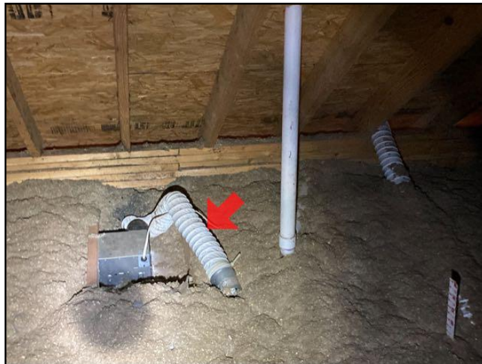
138. Fan exhaust tube detached
