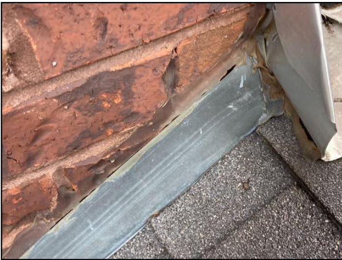
1. Caulking gaps at front sidewall flashing
