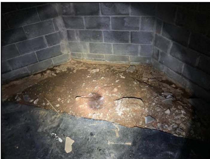
54. Vapor barrier missing
