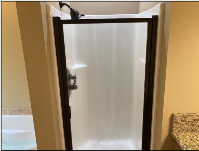
134. Shower is functional
