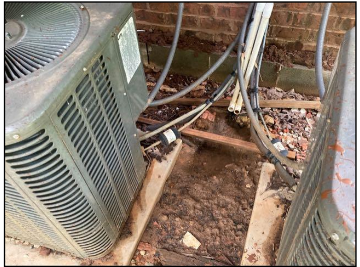
104. Condensate discharge location
