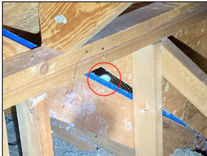
18. Hole in soffit
