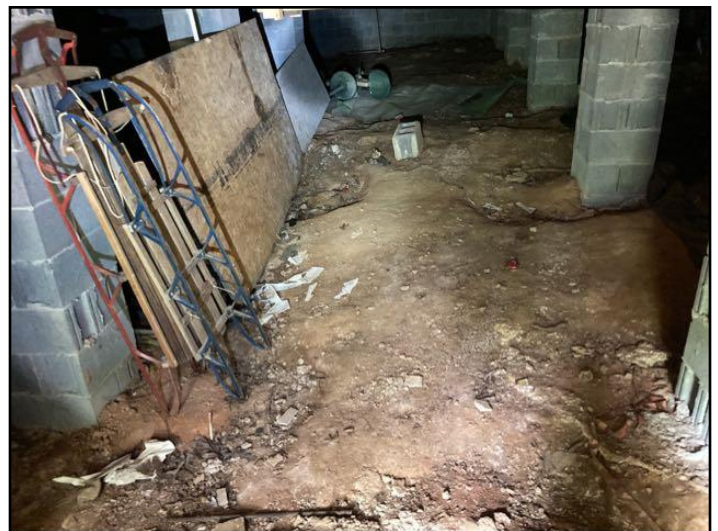
51. Vapor barrier missing
