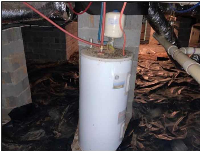
112. View of water heater
