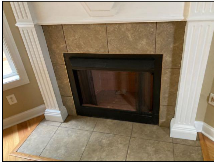
94. Gas logs not installed
