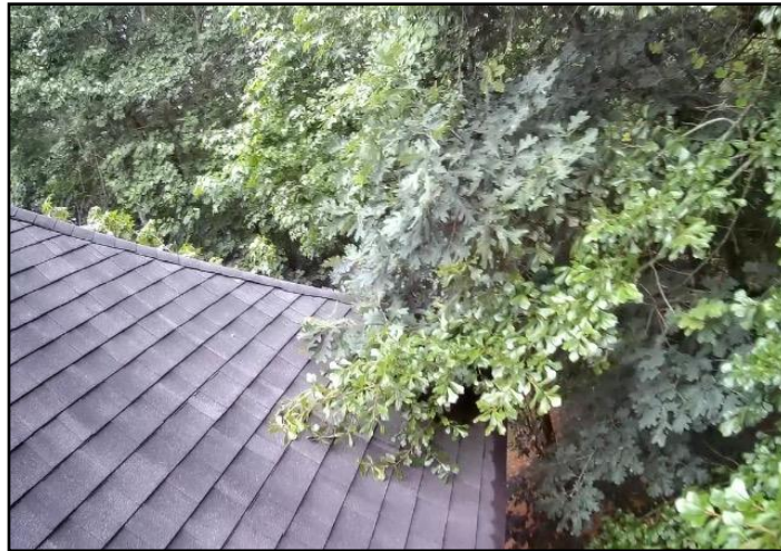
15. Tree branch/ roof contact
