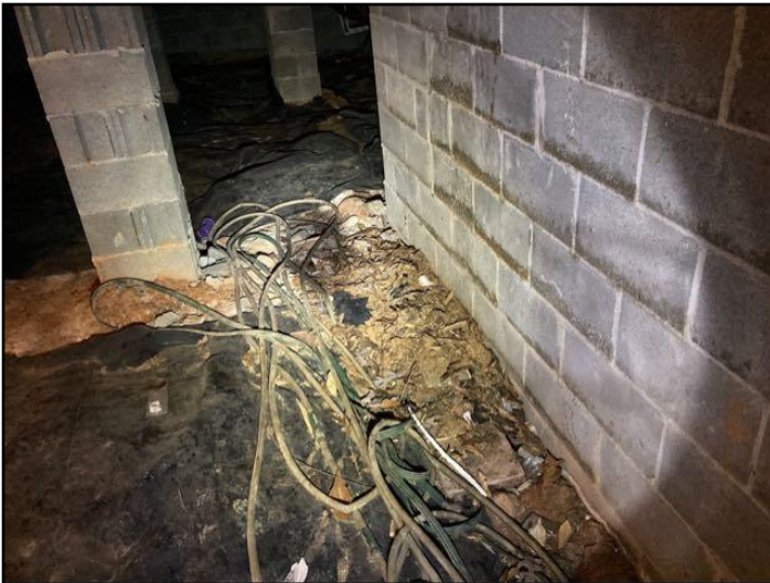
62. Debris under rear door
