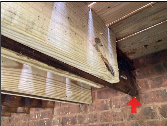
28. Sandwich repair not possible at bearing point
