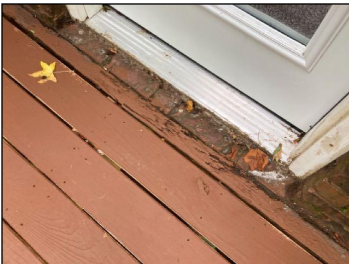
42. Rot/damage at deck edges
