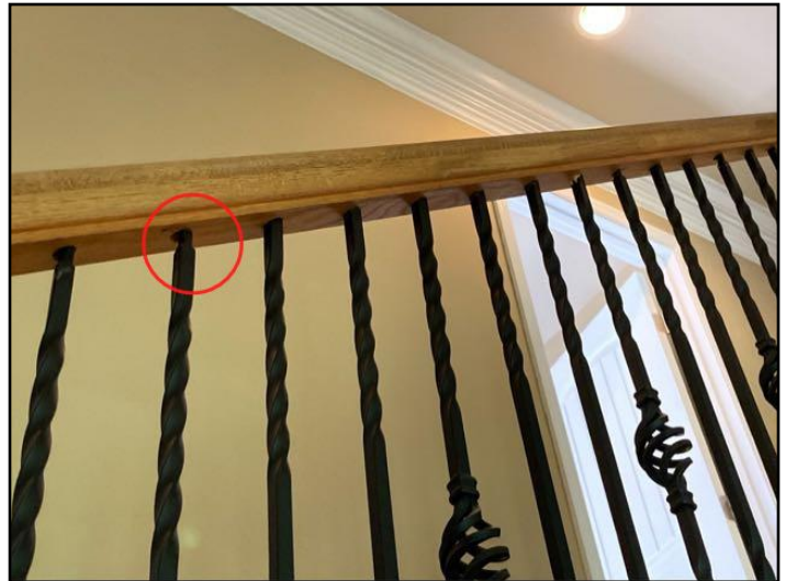
125. Rail baluster out-of-place
