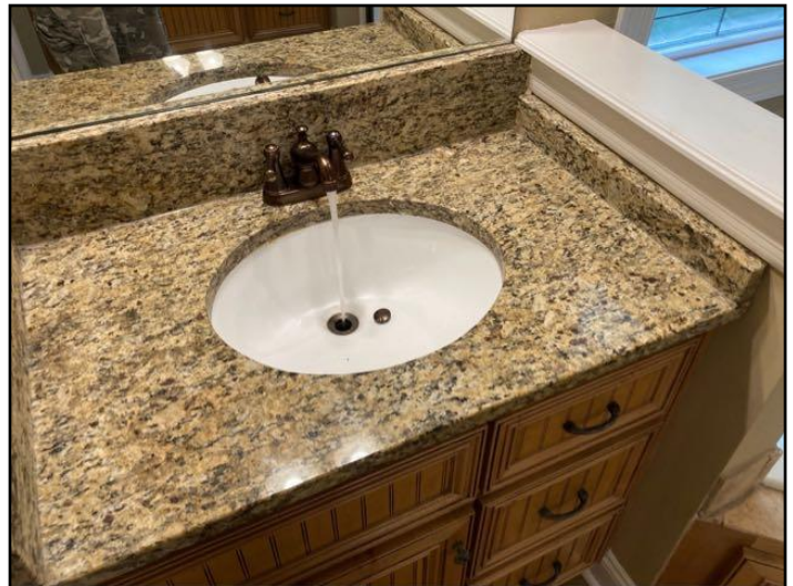
130. Sink is functional
