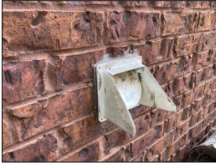
123. Damaged vent cover
