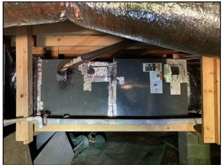
80. HVAC air handler (lower)
