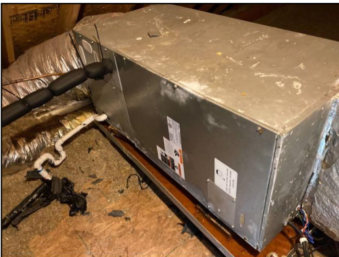
77. HVAC air handler (upper)
