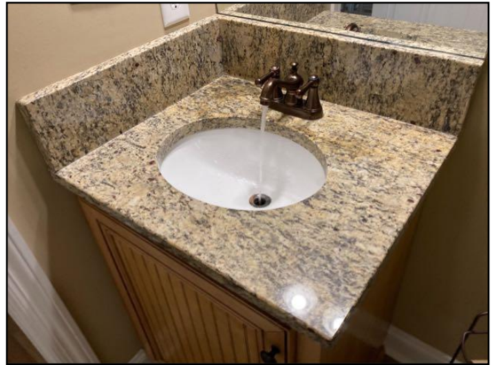
132. Sink is functional
