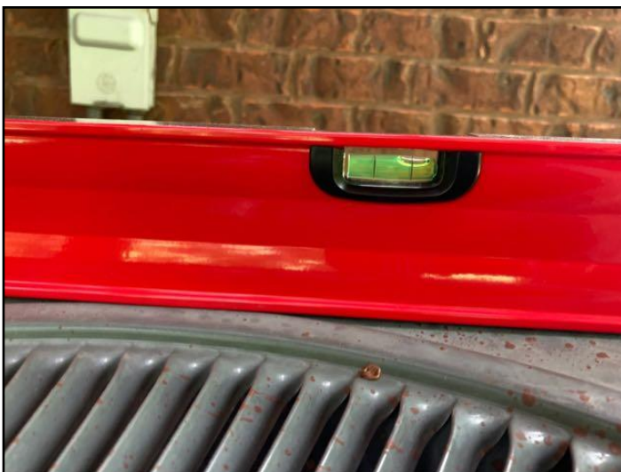
97. Condenser not level
