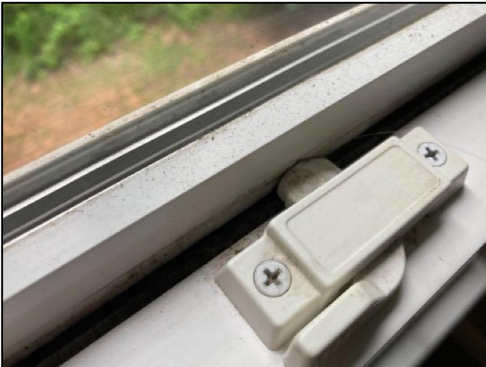
116. Lock not aligned
