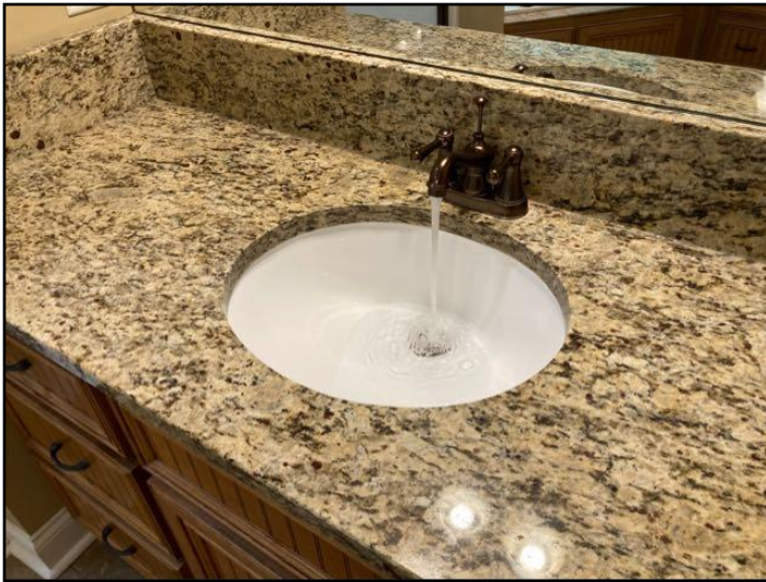
131. Sink is functional
