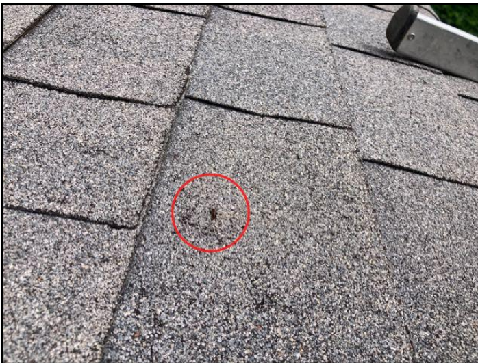
3. Nail pop at front center
