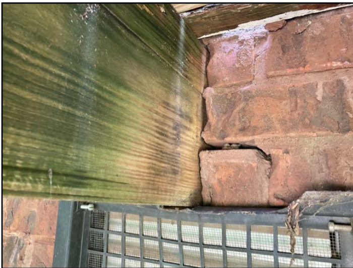
23. Loose brick at rear
