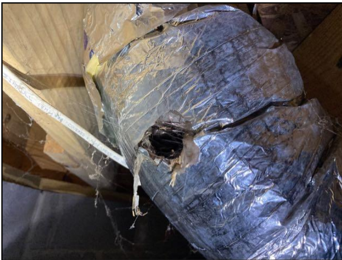
84. Rodent tunnel in duct
