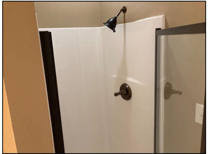
135. Shower is functional
