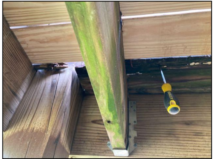
37. Rot/damage at deck edges
