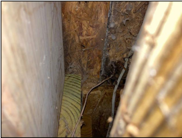
64. Stains/ wood damage under living room door
