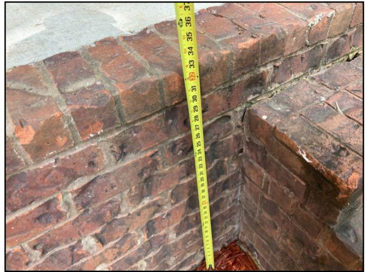
48. Porch height requires guardrail
