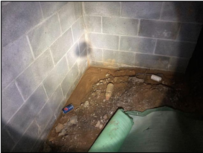
52. Vapor barrier missing
