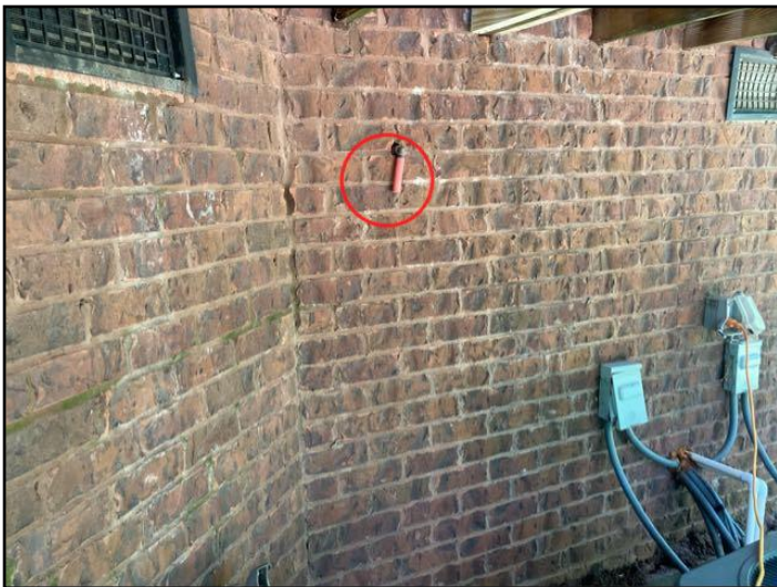
111. Improper discharge location/height
