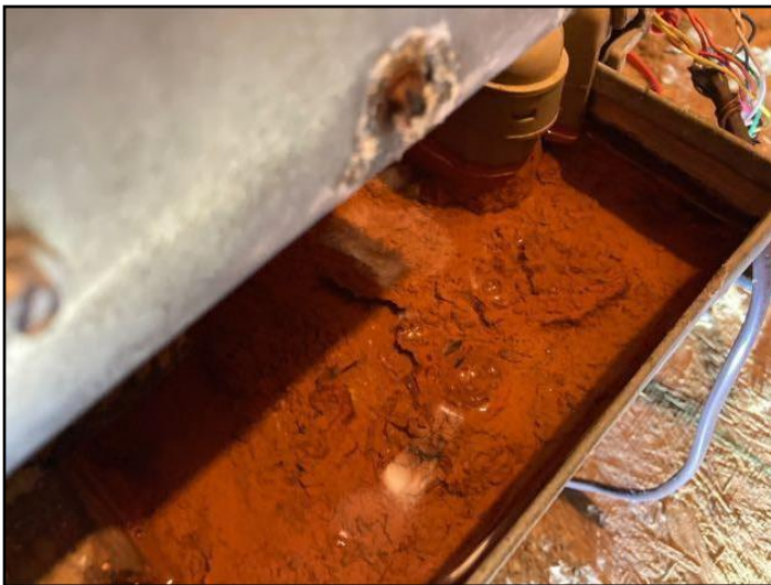
79. Water/rust in pan
