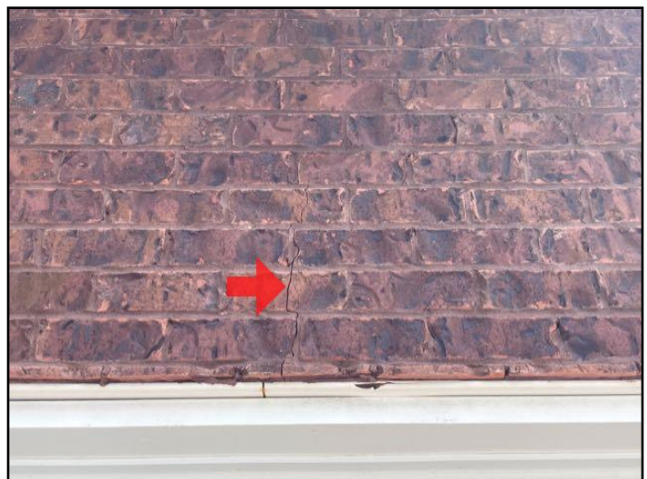
22. Brick veneer crack above garage door
