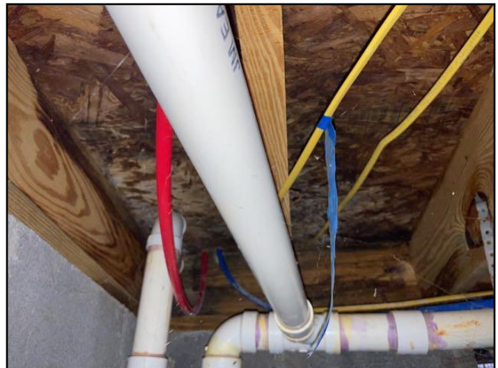
71. Large water stain under laundry room
