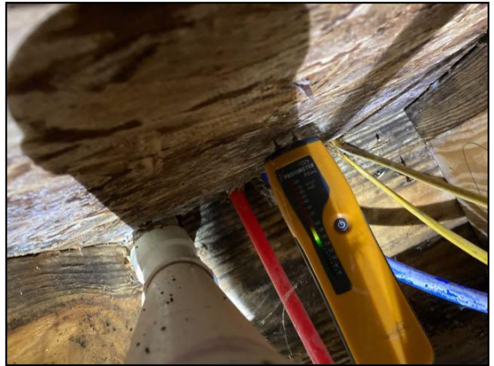
73. Acceptable moisture content under laundry
