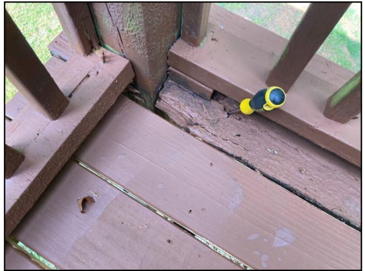
41. Rot/damage at deck edges
