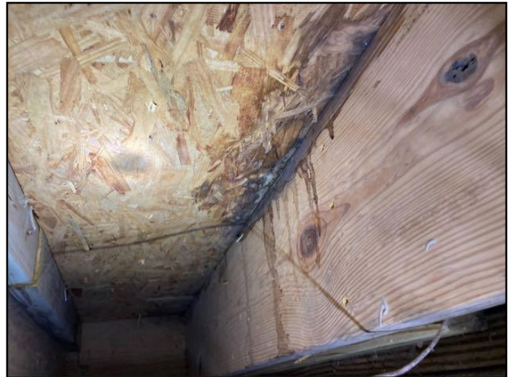
63. Water stains under rear living room door
