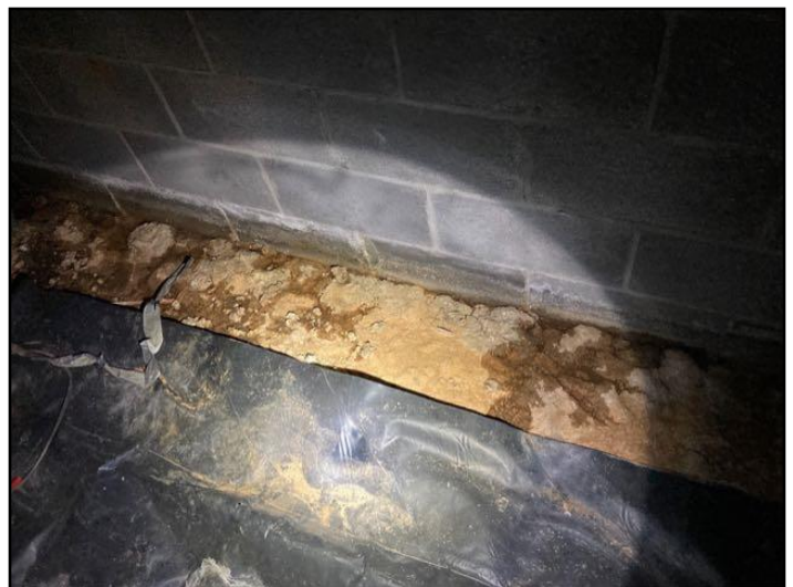
55. Water seepage at left side
