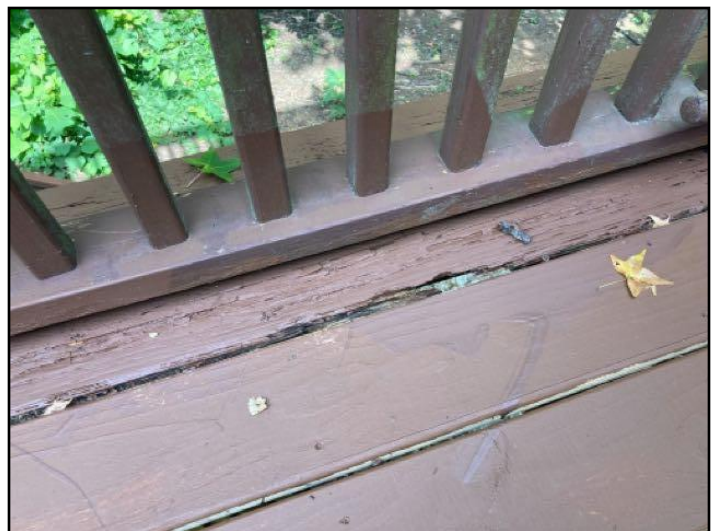
43. Rot/damage at deck edges
