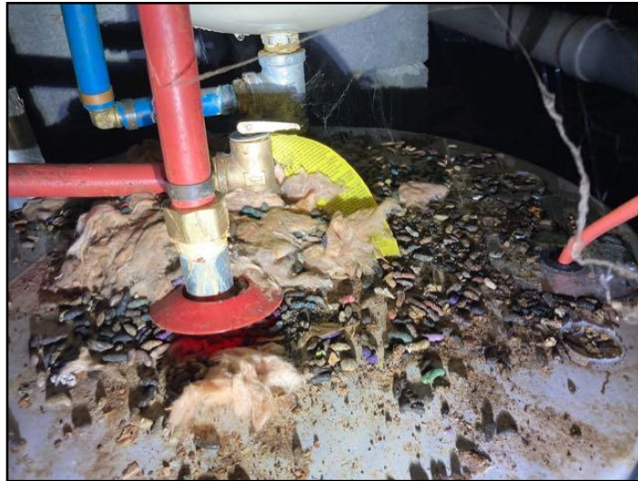
126. Rodent droppings on water heater (crawlspace)
